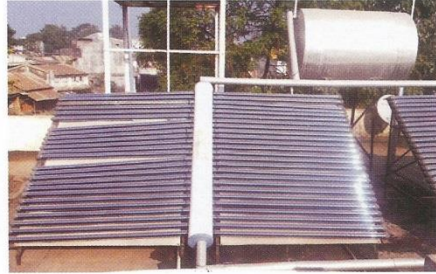
Solar water heater
