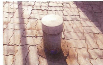
Water Recharge Borewell
