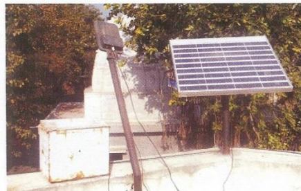
Solar street light
