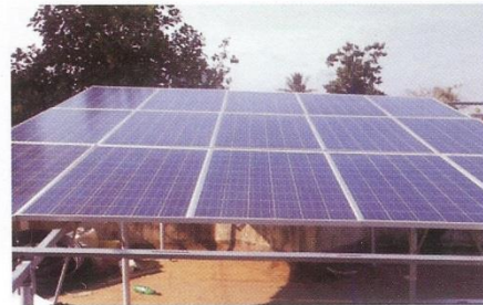
Solar Electricity generation 18 Kw
